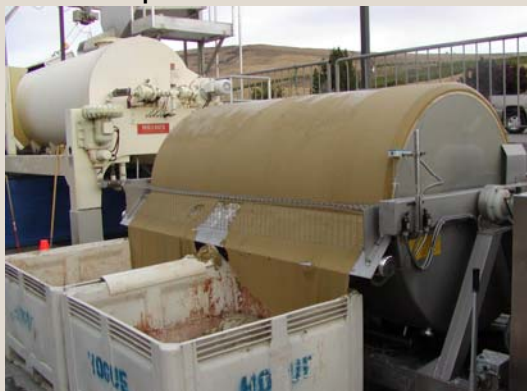
Spent DE Removal
